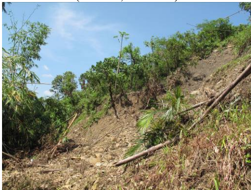
(c) 坡趾受溪溝侵蝕而崩滑 (206961, 2550258)
